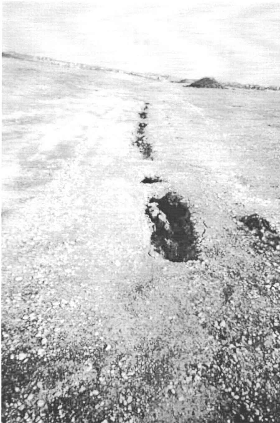
Fig. 4 Post construction settlement of utility trench backfill.
