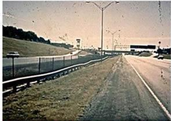
Guardrail between pavement lanes on expansive clay subgrade IH37, San Antonio, Texas (c. 1974)
