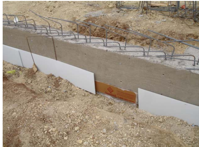
Example of Soil Retainers adjacent to Carton Forms placed under grade beams
