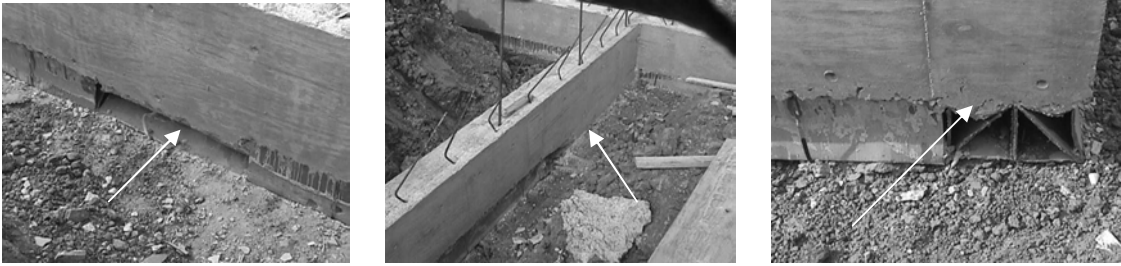
View of failed boxes
