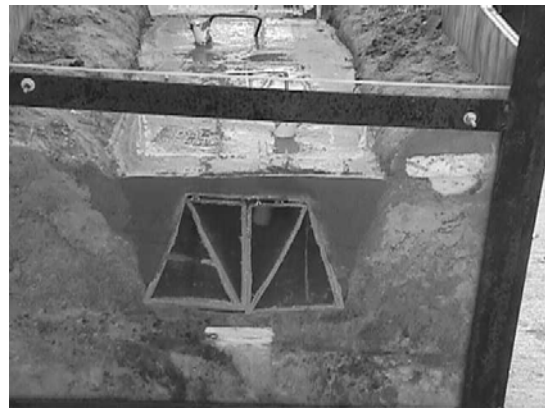
View of beam void box with retainers
